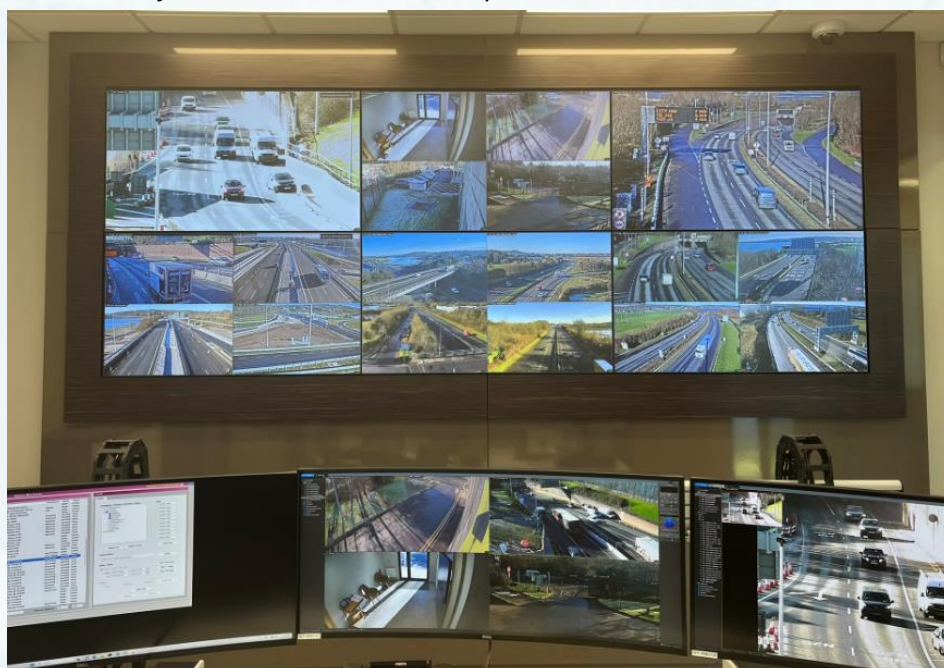
JLT Control Room Video Wall
